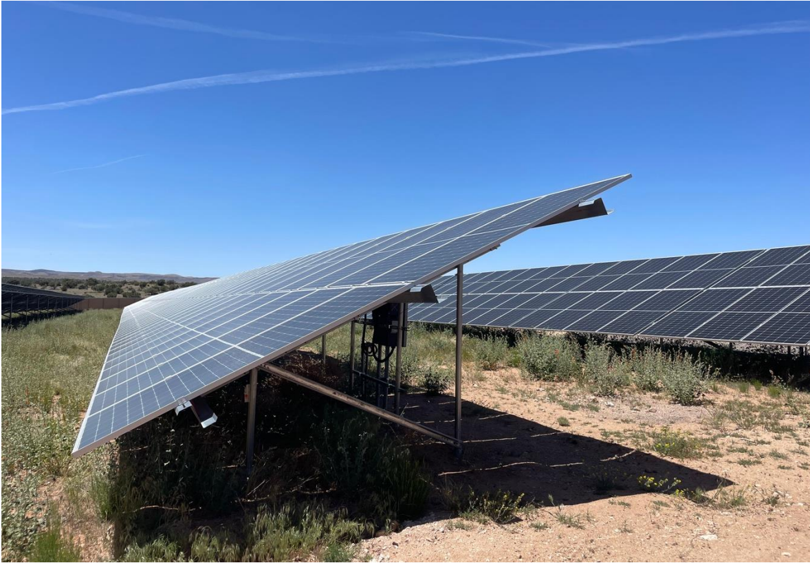
Example of a south facing fixed-tilt solar array (Photo credit: Laura Beshilas, NREL)
