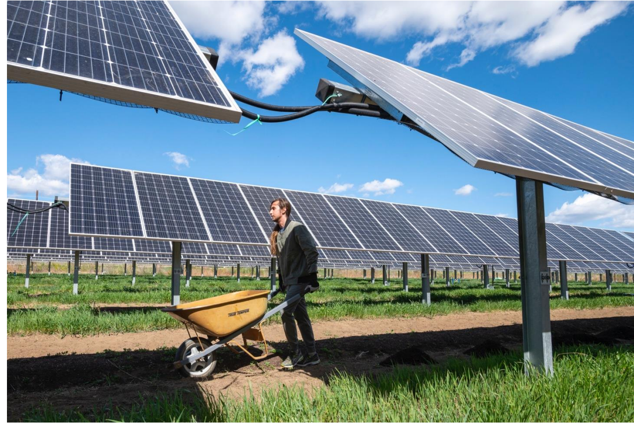
An example of overhead wire management at Jack's Solar Garden (Photo credit: Bryan Bechtold / NREL)
