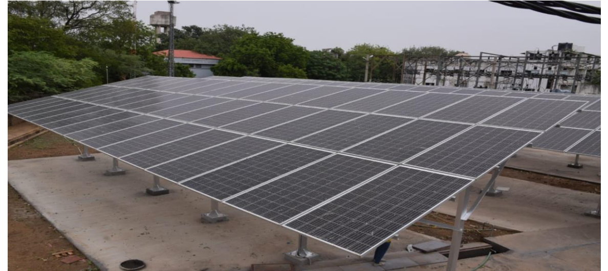
100 kWp Solar PV Carport
