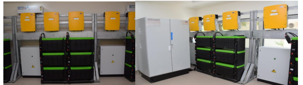
Sunny Island Inverters & Battery Clusters
