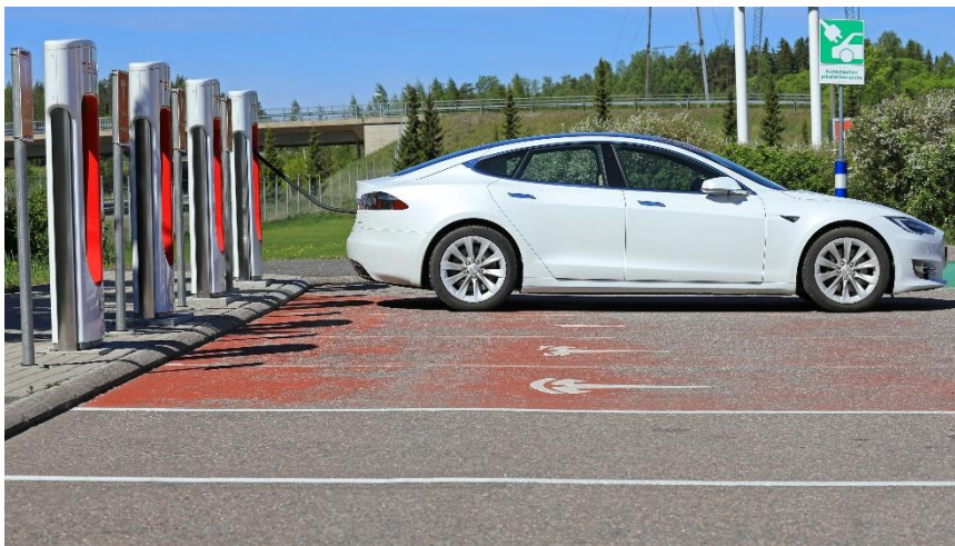
FIGURE 3-40: AN OUTDOOR CHARGING STATION
