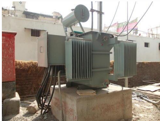
FIGURE 3-38: PLINTH MOUNTED DISTRIBUTION TRANSFORMER
