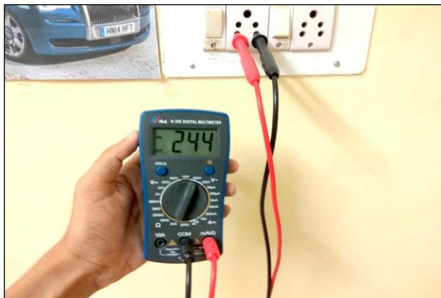
FIGURE 5-4: USING A MULTIMETER TO CHECK THE PHASE TO NEUTRAL VOLTAGE
