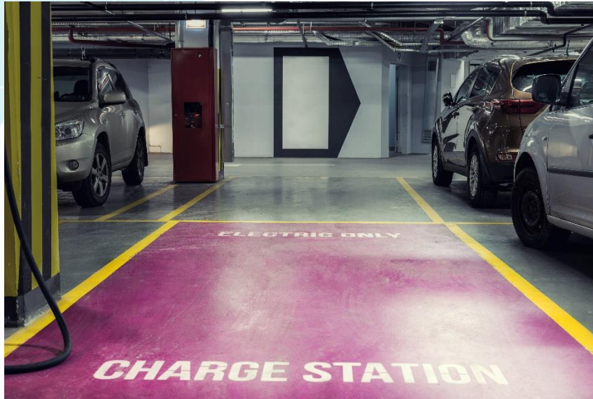
FIGURE 3-41: AN INDOOR CHARGING STATION
