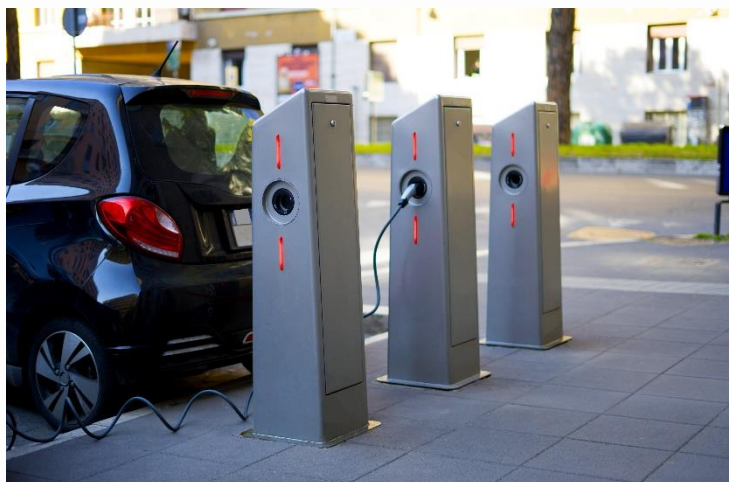
FIGURE 3-36: ELECTRIC VEHICLES PARKED FOR CHARGING
