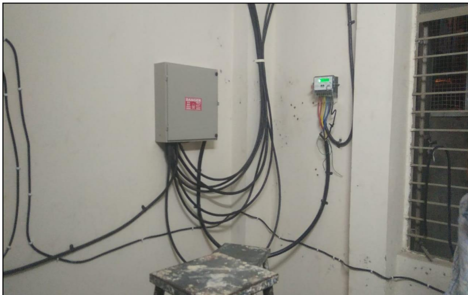
FIGURE 4-14: IMPROPERLY DRESSED ELECTRICAL WIRING
