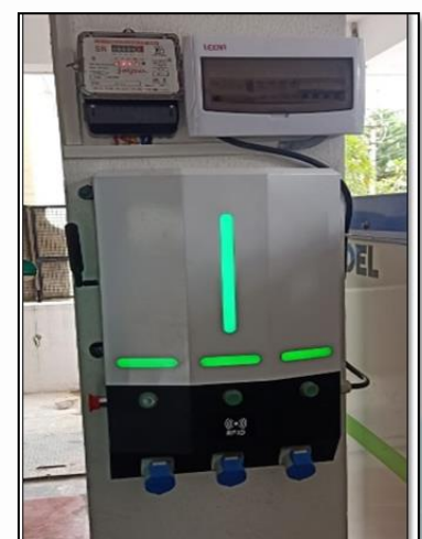
FIGURE 4-9: A 10 KW AC CHARGER ON A SHARED CONNECTION, CONNECTED THROUGH A SUBMETER
