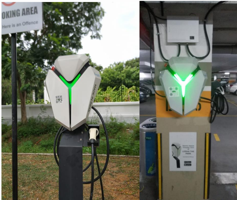
FIGURE 3-42: A WALL AND PEDESTAL MOUNTED EV CHARGER
