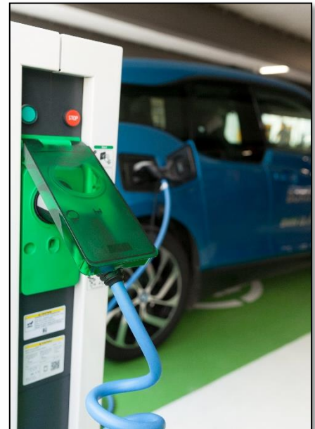
FIGURE 4-8: A DC CHARGER ON ITS DEDICATED CONNECTION
