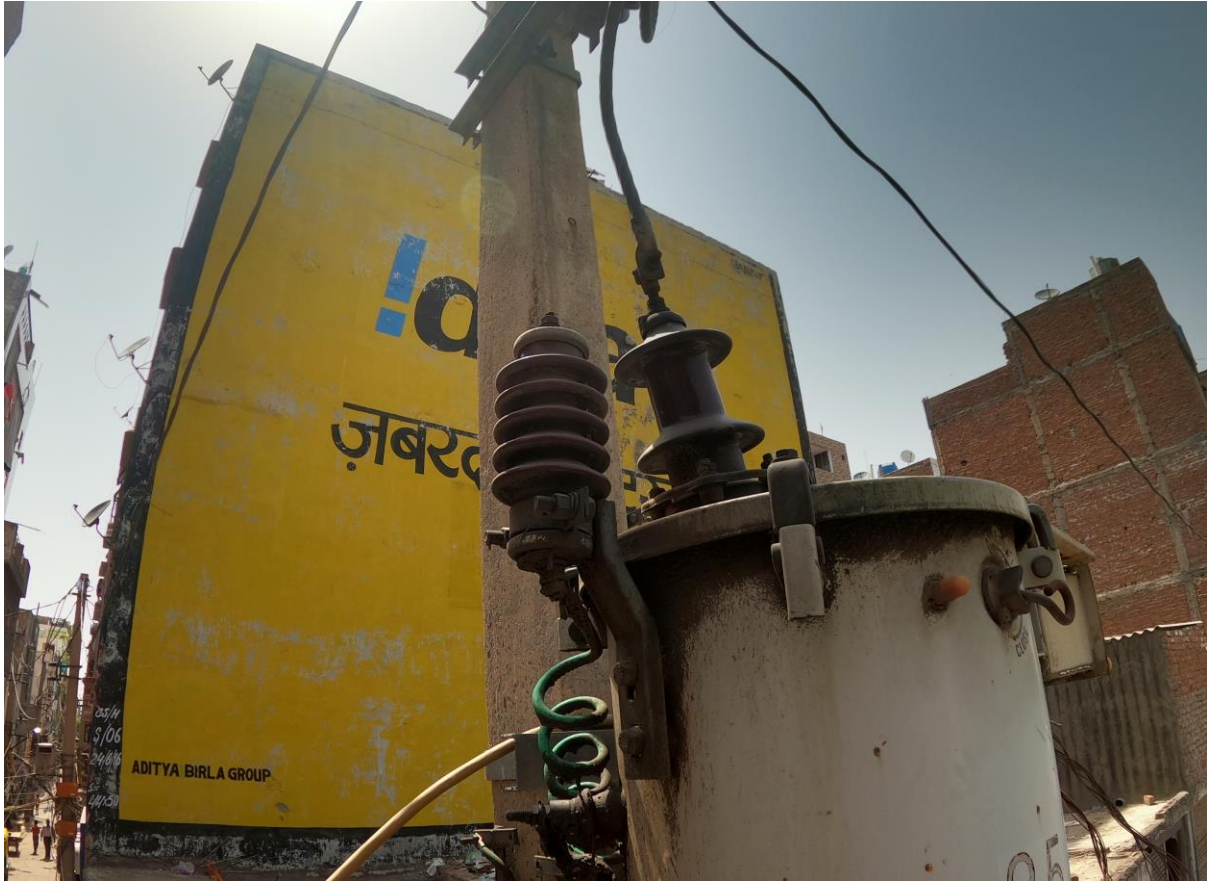
Figure 5: Missing fuse and earthing failure in DT
