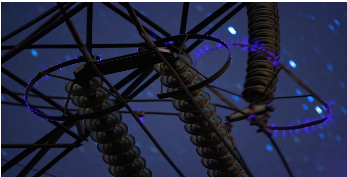
Figure 23: Corona discharge on an insulator of a high-voltage line
