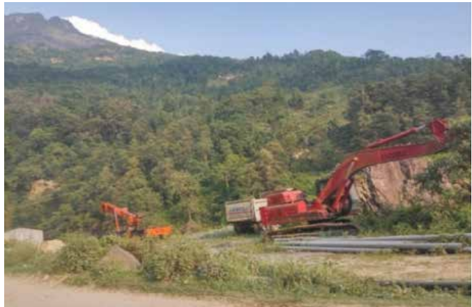
Abandoned equipment belonging to former contractor IVRCL at Galeshwor
