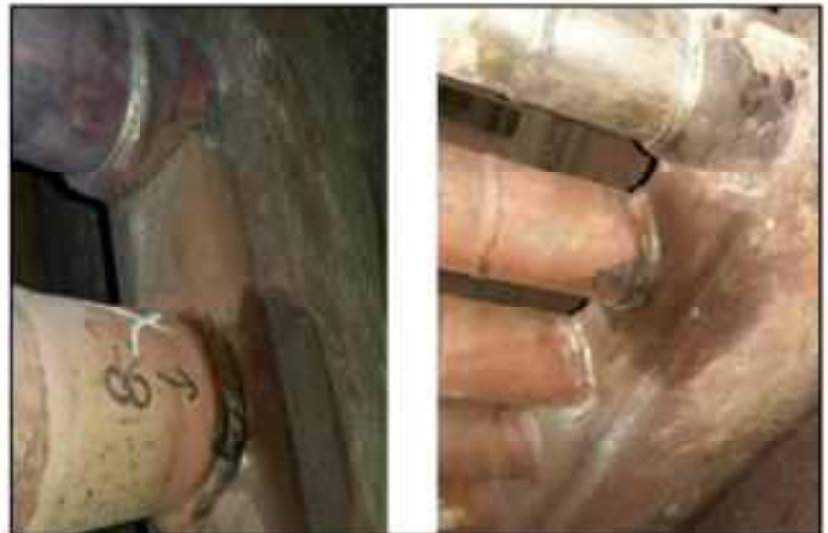
Figure 16: Attachment weld failure
