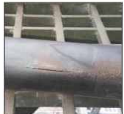
Figure 11: SH tube longitudinal crack
