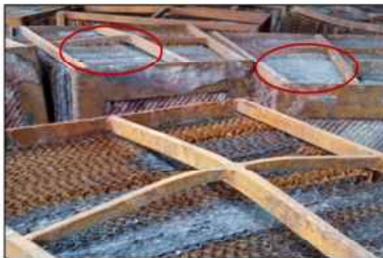
Figure 29: Partially choked APH baskets (removed after water washing)
