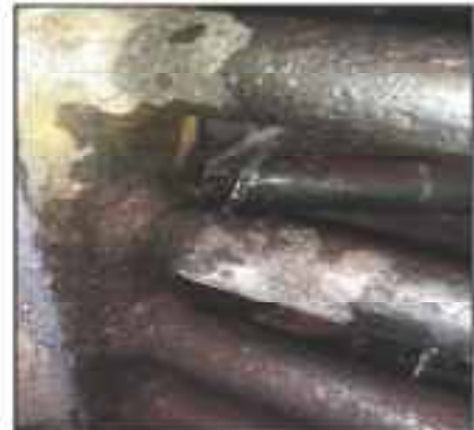
Figure 7 (a) SH Stub joint crack
