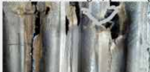
Figure 61: Second pass hanger tube erosion
