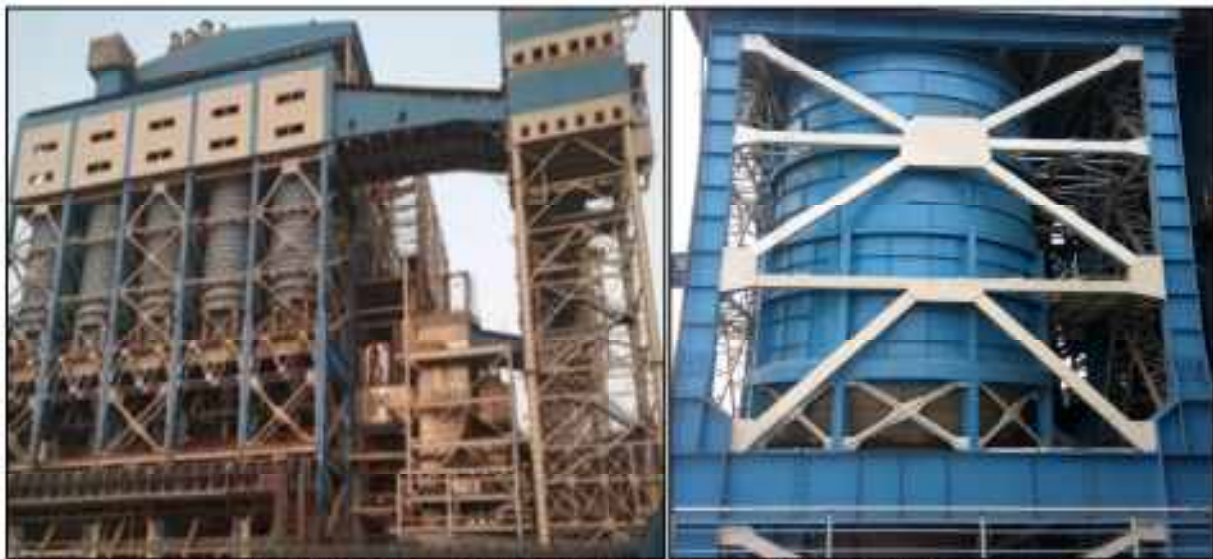
Figure 62: Coal bunkers must be emptied when unit is under long shutdown
