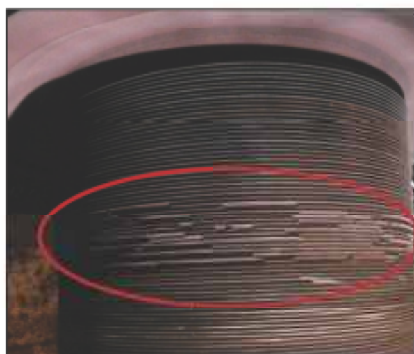
Figure 23: Damaged Turbine sealing
