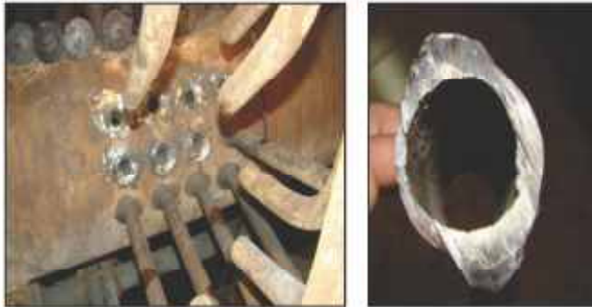
Figure 25: FAC- Economizer inlet stab joint pipes thickness is reduced
