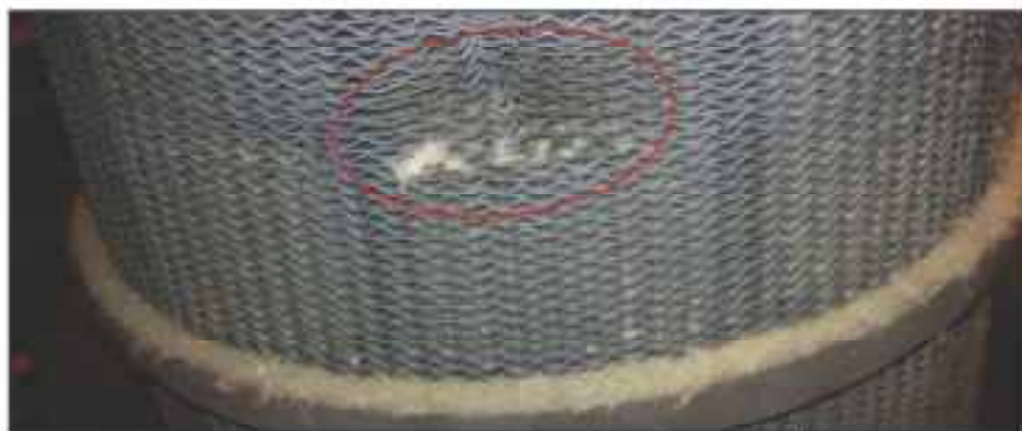
Figure 19: Damaged Strainer (MS Line)
