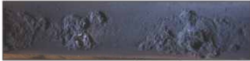
Figure 24: Water side corrosion
