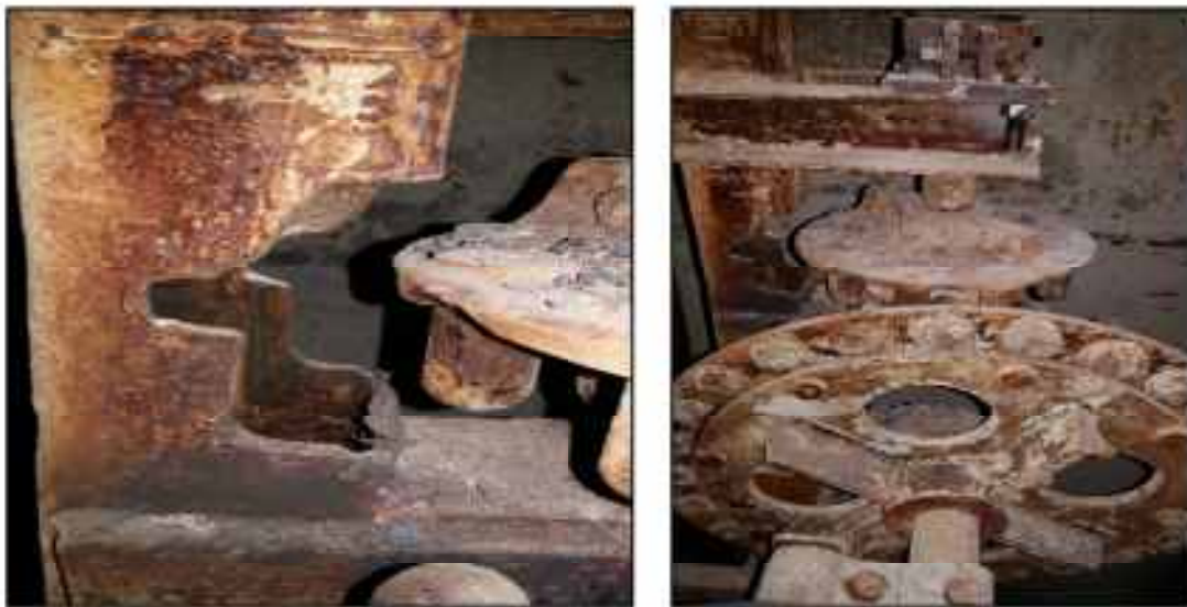
Figure 30: Corroded ESP Internals
