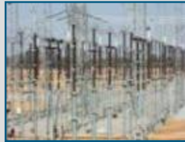
Air Insulated Switchgears
