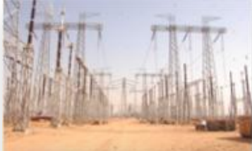
Commissioned 765 kV s/s for PGCIL at Bhiwani in 2012
