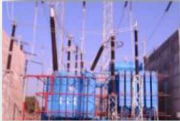
Commissioned the first fully integrated 765 kV transformer at Vadodara, India for LANCO – Anpara “C” in 2011
