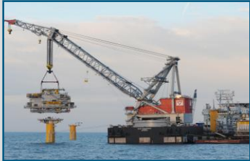
Electrical substations, Turnkey solutions & Services
