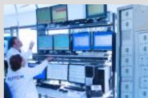
Substation Automation Solutions
