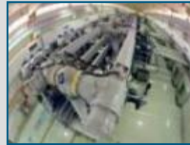
Gas Insulated Switchgears
