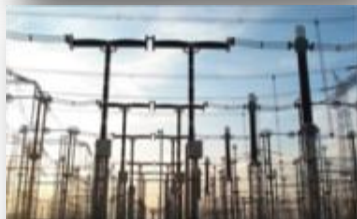
India's first 765 kV AIS substation Project for NTPC Sipat (19 Bays) in 2009
