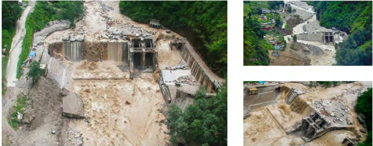
Figure 3. Damage to Nepal's Upper Bhoite Koshi hydropower plant after a 2016 glacial lake outburst flood caused by a heavy rainfall event.
