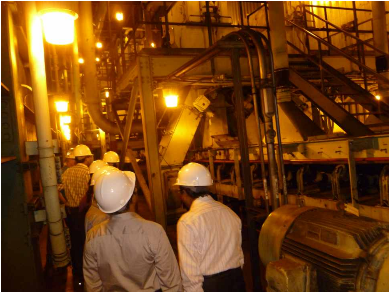
USAID PACE-D TA Program Study Tour to U.S. in July 2013: Coal Tripper Deck at OUC Stanton Energy Center.
