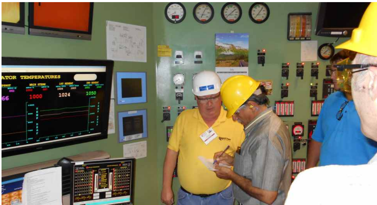
USAID PACE-D TA Program Study Tour to U.S. in July 2013: Control Room at AEP Amos.
