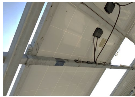
D. Improper cable management (no name tags to identify the cable)
