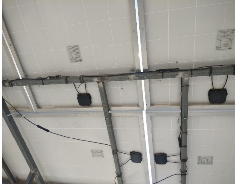
A. Indicating good cable management practice
