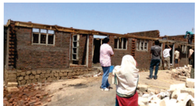
Construction of a low-income home in Jasdan, India that will receive a cool surface exterior
