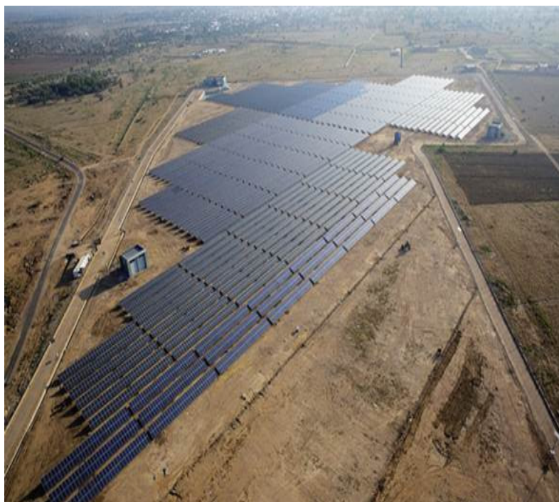
OPIC and Ex-Im Bank will support large solar projects such as the 5 MW grid connected solar power plant at Khimsar village, Rajasthan.
