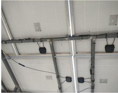
A. Indicating good cable management practice
