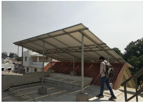
C. Inaccessible array. Notice how the lower end of the module tips dangerously into the slope
