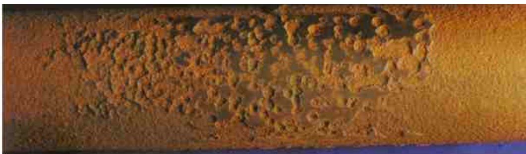
Figure 9-33: Acid Dewpoint Corrosion
