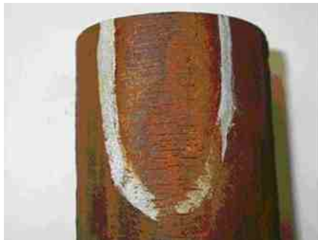
Figure 9-37: Supercritical Waterwall Cracking
