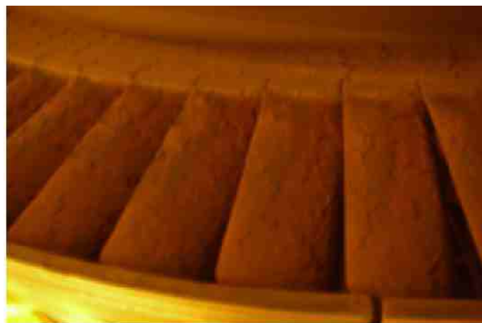
Figure 5-9: Turbine Iron & Silica Deposits
