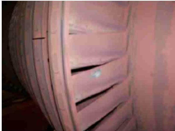
Figure 5-10: Turbine Iron Deposits
