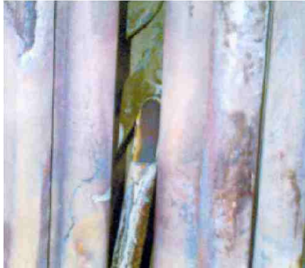
Figure 5-4: Corrosion Fatigue Tube Failure
