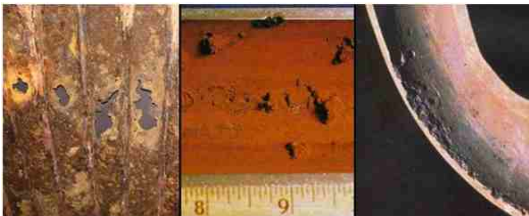
Figure 9-46: ID Oxygen Pitting Corrosion
