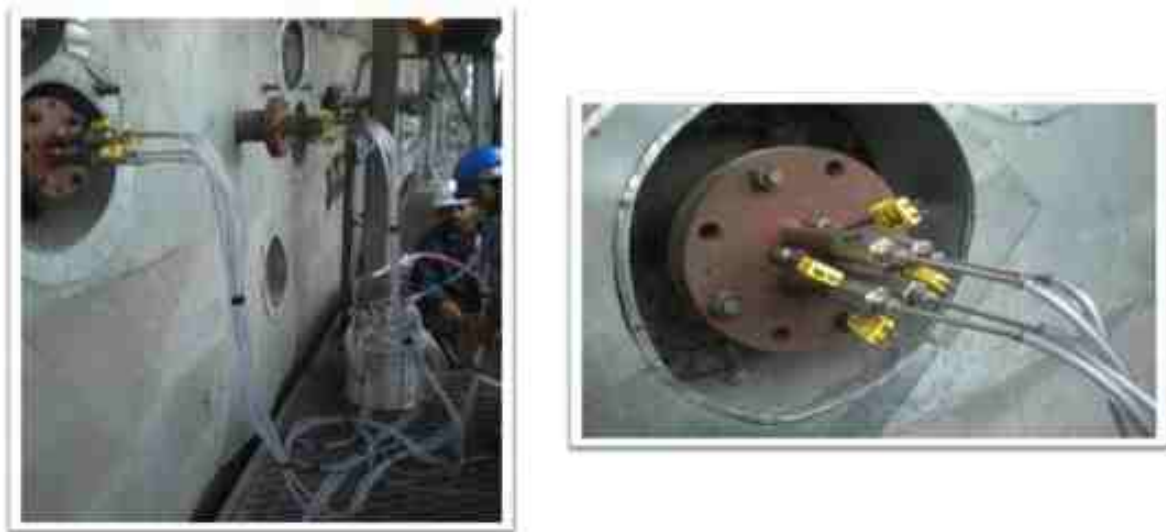
Figure 6-29: Photograph - Multi-Point Sampling Probes
